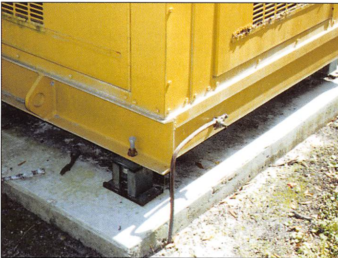
Figure 6. The emergency generator is also connected to the ring-ground, and is additionally grounded to reinforcing rods in its concrete pad.
