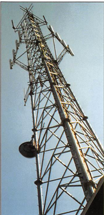
Figure 1. The Communication Center shares its 90-ft antenna tower with a cellular telephone/long-distance service provider. Both tenants maintain their own lightning protection/grounding systems. Of the two systems, the Communication Center's is far more extensive and considerably more robust.
