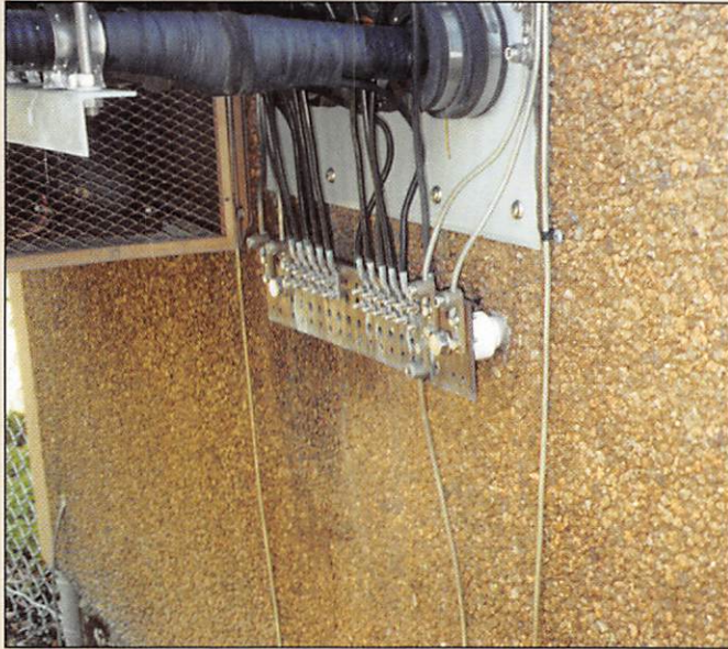
Figure 12. Grounding connections to coax cable shields at the cellular-telephone/long-distance service provider that shares Winter Park's antenna tower are made on the horizontal run of the cables. Connection to vertical runs provide better lightning protection, according to PSI's John West. #2 AWG grounding electrode conductors installed by the telephone company are the minimum size permitted under the NEC. The Winter Park Communication Center up-sized its grounding electrode conductors to more-robust 4/0 copper.
