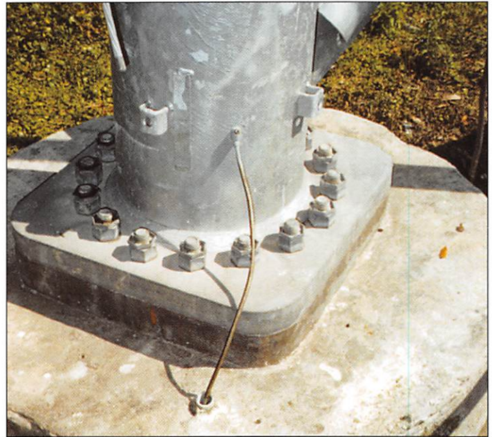
Figure 4. The antenna tower was grounded during construction using #2 AWG bare copper bonded to reinforcing rods in the footers (Ufer grounds). PSI augmented this system by bonding each of the tower's four legs to two electrodes (not shown) driven on diagonals extending outward from the tower. The new grounding-electrode conductors are bare 4/0 copper.
