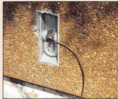
Figure 13. Grounding connection to a lifting lug on the telephone provider's modular building. There is no assurance that the lifting lug is actually bonded to the structure's metal frame.
