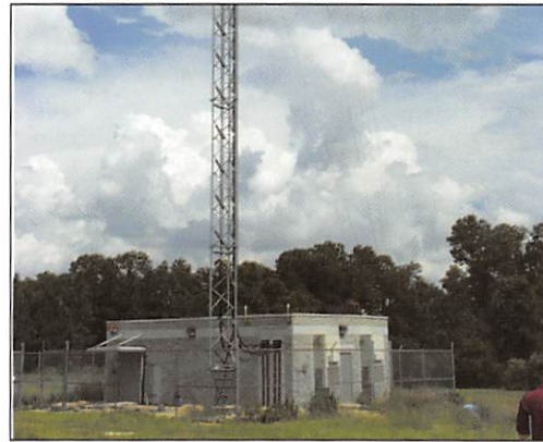
Figure 15. Reedy Creek, one of Orange County's two remote repeater sites, is underlain by high-resistivity "sugar sand." Poor soil conditions, along with neglected chemical-type electrodes, raised the site's ground resistance to more than 1,000 ohms.
