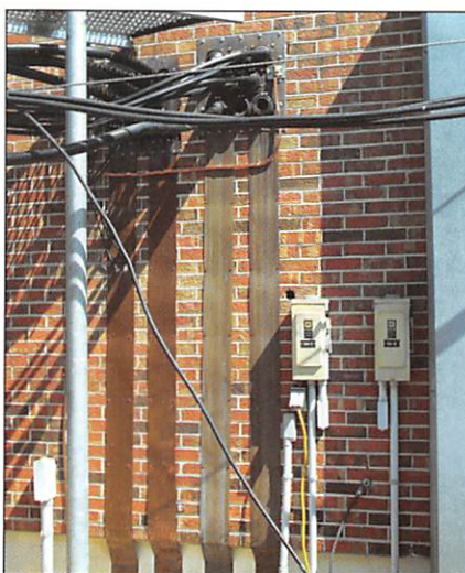
Figure 4. Only one of the four copper strips shown leading from the site's two antenna cable firewalls was actually connected to the counterpoise. The other three were simply buried. The copper strips are now augmented with AWG 4/0 copper securely bonded to the firewalls and to the new grounding electrode.
