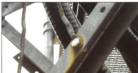
Figure 11. Corrosion raised resistance at an existing cable shield ground connection on the Clarcona tower.
