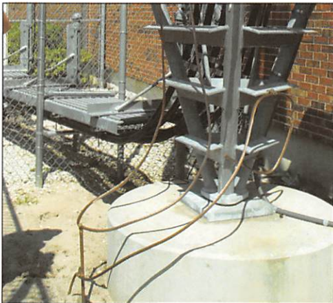
Figure 2. Bare AWG 4/0 copper conductors are exothermically bonded to a new 60-ft (18-m) grounding electrode at the Apopka tower base (lower left) replacing the all-thread rod. Resistance to earth is 4.3 ohms.
