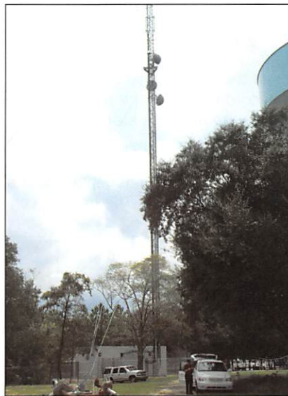
Figure 10. Like the Apopka hub, Orange County's smaller Clarcona site suffered from high ground resistance, inadequately maintained chemical electrodes, poor bonding and ungrounded equipment cabinets. Upgrades include a new 60-ft (18-m) deep electrode with less than 5 ohms resistance, firm bonding of all connections, installation of heavy copper grounding conductors to all equipment cabinets plus new halo grounds in the comm room.
