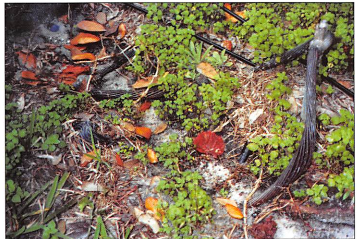
Figure 2. One of numerous grounding electrode conductors installed by PSI at Resort World. The 4/0 conductor at right leads to six 50-ft (15-m), 3/4-in (19-mm) diameter copper-clad rods set in a row running parallel to the rear of the resort's communications and computer offices, about 12 ft (4 m) from the structure. The conductor leading to the left tags onto one of the building's original 10-ft (3-m) electrodes. In accordance with PSI specifications, ground resistance of all new electrodes is less than five ohms.
