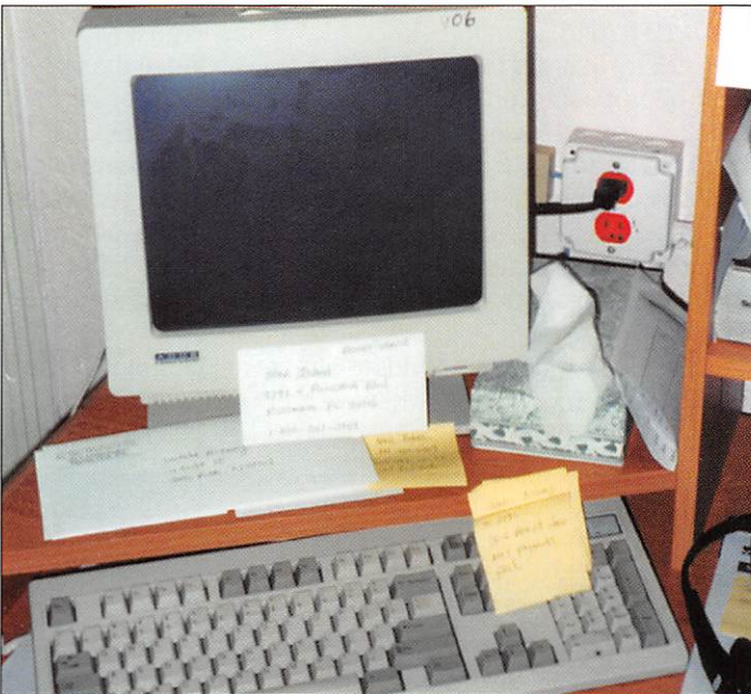
Figure 7. A typical workstation in the construction office that technicians at Resort World call "Hell House" for its many power quality-related problems. The problems are a thing of the past, since PSI installed grounding electrodes having less than 4 ohms ground resistance, plus TVSS protection and dedicated circuits for sensitive electronic equipment. In addition, PSI specified isolated grounds for the sensitive circuits, as can be seen by the orange-colored outlet shown in the photo. Finally, PSI specified that branch circuits serving sensitive electronic equipment must contain no more than two outlets each. Among other benefits, limiting the number of outlets per circuit reduces the magnitude of harmonic currents on neutral conductors.
