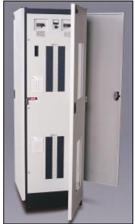
RPP systems are available in many different configurations. The front view of the RPP system shown above provides the user 84 poles of 60 Hz distribution capacity.
